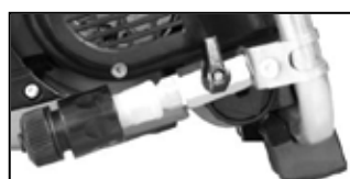
water supply closed (valve lever across)
